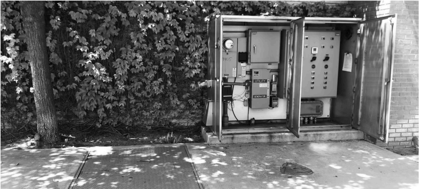
Carmenita Sewer Lift Station
